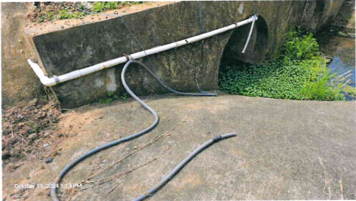
Imagen1: Vandalismo ocasionado a ITS DAI-28
